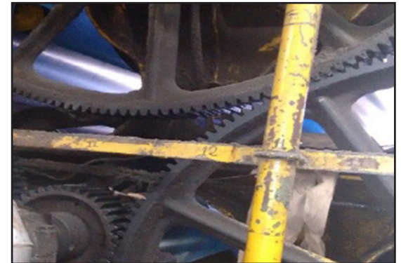
Clean and quiet operation of the timing gears.
